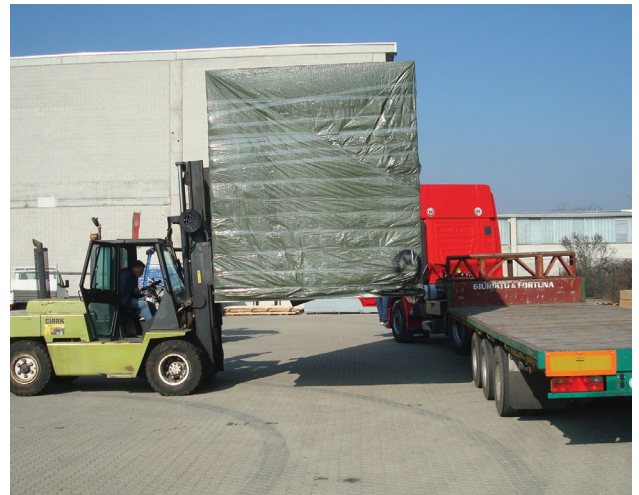
An ICE Cube Air modular data center is unloaded as part of the Installation & Commissioning service.
