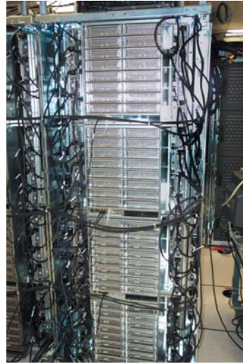
Figure 4: Multiple SGI Altix ICE Racks, Reduced Cabling
