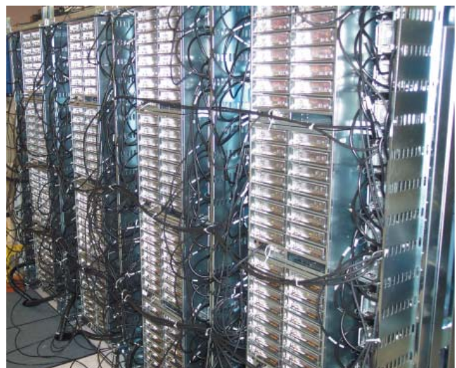
Multiple SGI Altix ICE Racks, Reduced Cabling
