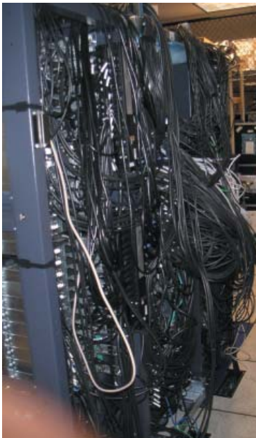
Traditional Cluster Cabling
