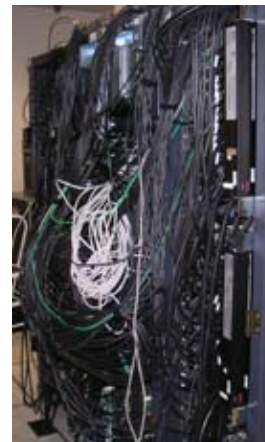
Traditional cluster cabling
