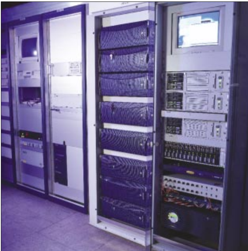
Four SGI Media Servers for broadcast (purple rackmounted systems), and RAID-3 storage by Ciprico provide dual redundant systems for newsroom and airplay operations at Danish Broadcasting.
